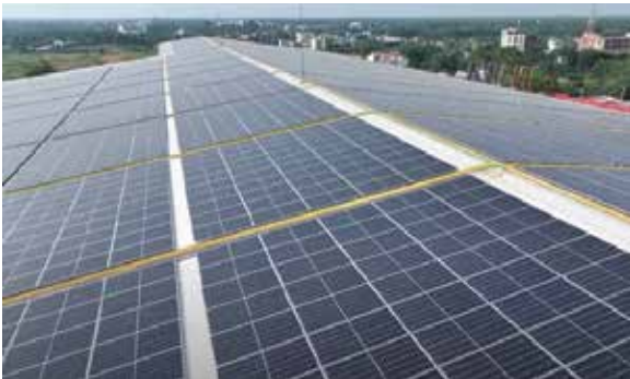
Image of 2.2 MW capacity Solar Panel Installation.
